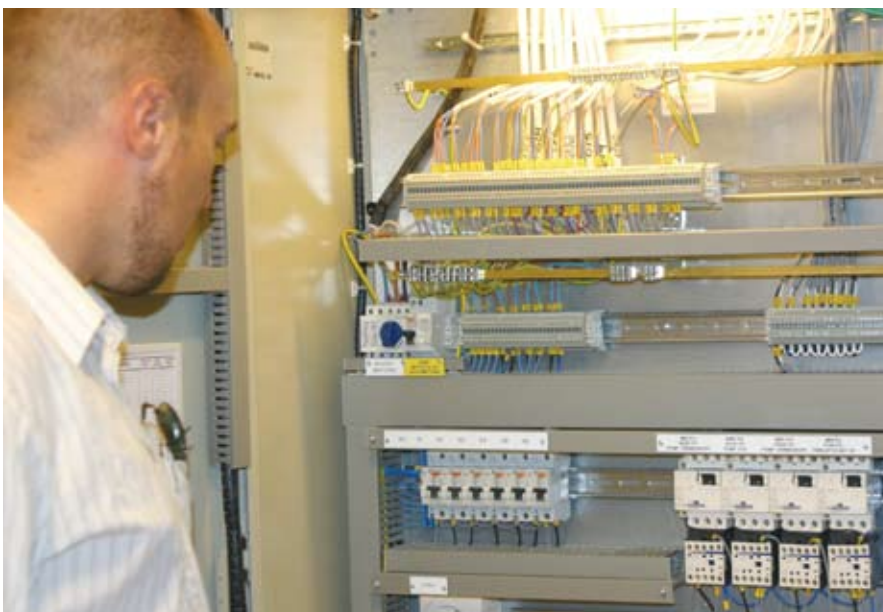
Input from room devices is handled by computerized regulators
